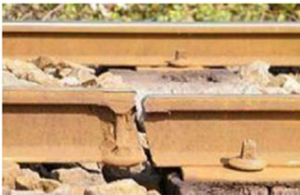
Figure 1: Crack On Railway Track
